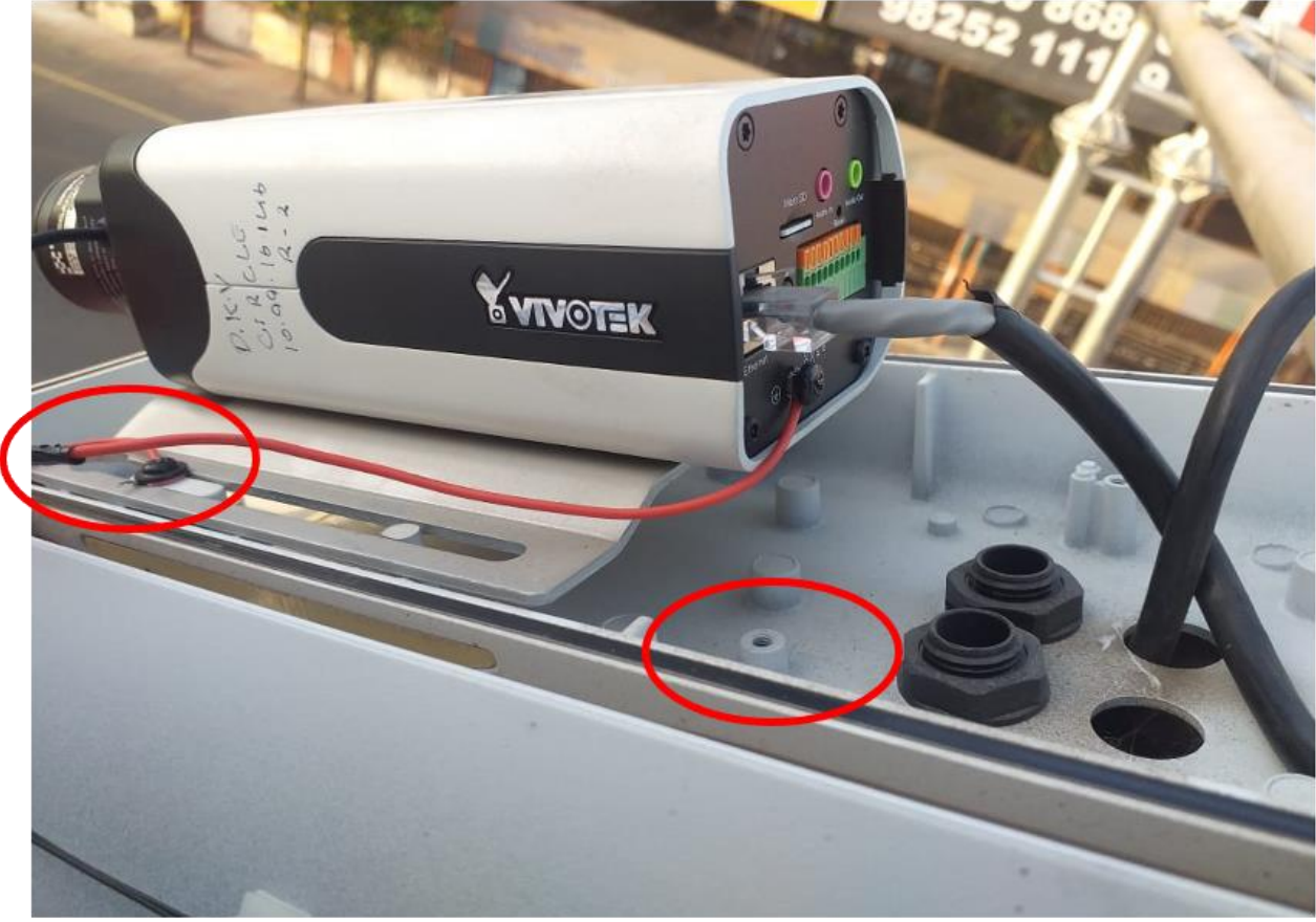
Incorrect grounding point
